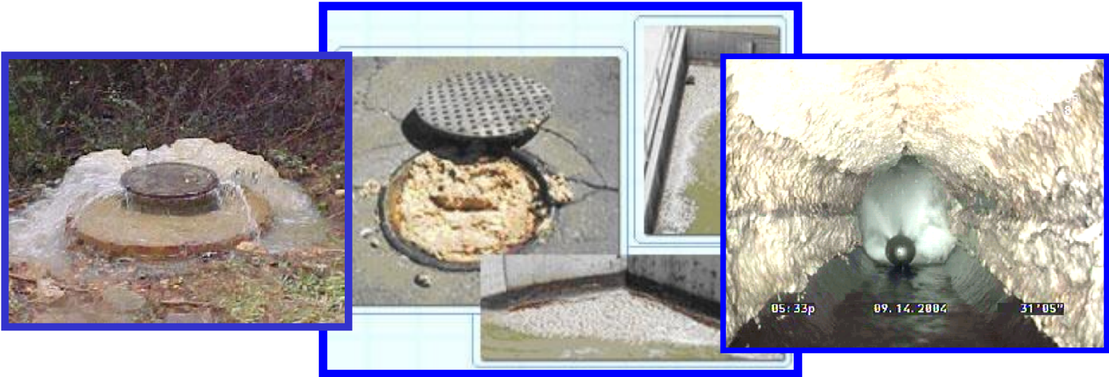
Figure: The effects of FOG accumulation in the sanitary sewer system.
